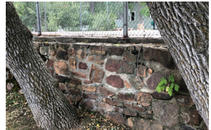
Figure 4: The retaining walls throughout the Chautauqua site are experiencing degrees of failure as increased water pressure, soil movement, and age are combining to threaten the stability of the walls.
