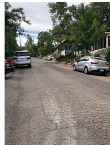
Figure 2: The road surfaces within the Chautauqua site are being damaged by heat and precipitation.
