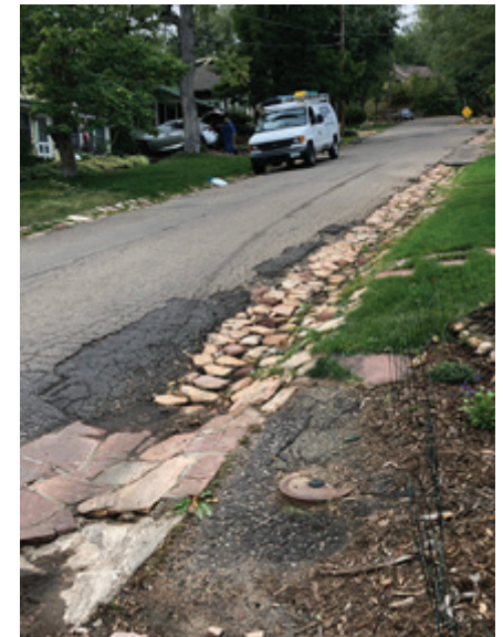
Figure 3 The Chautauqua site has a long history of battling water drainage issues with the historic stormwater system.
