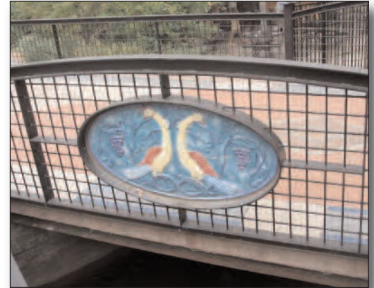
Art can be readily incorporated into functional elements, such as bridge railings, throughout the area.
