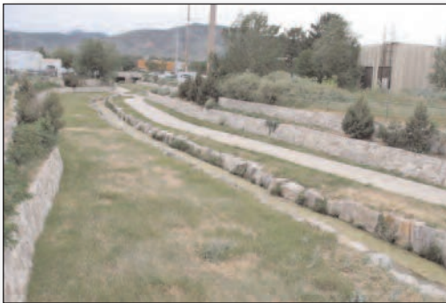
Today the Goose Creek channel between the rail tracks and 30th Street has a concrete liner and rock edging.
