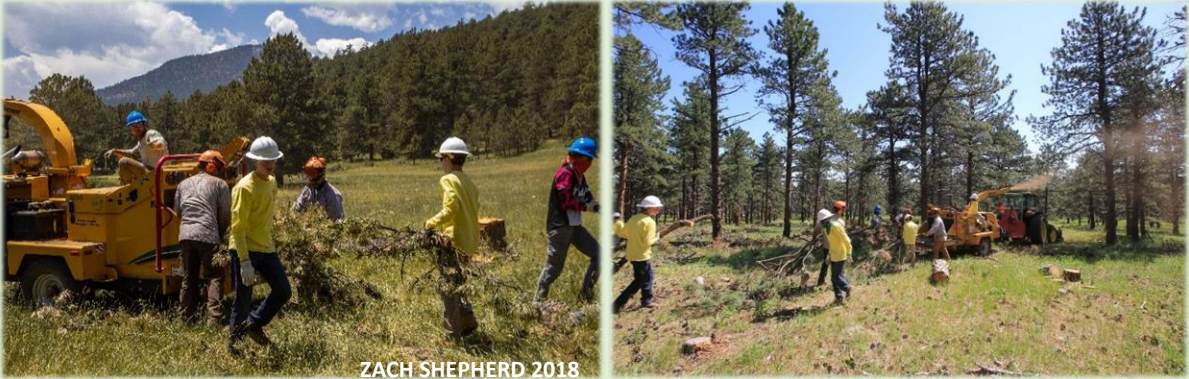
CREW 3 MOVING SLASH TO A CHIPPER AND DISPERSING FRESH MULCH ON THE LINDSAY PROPERTY.
