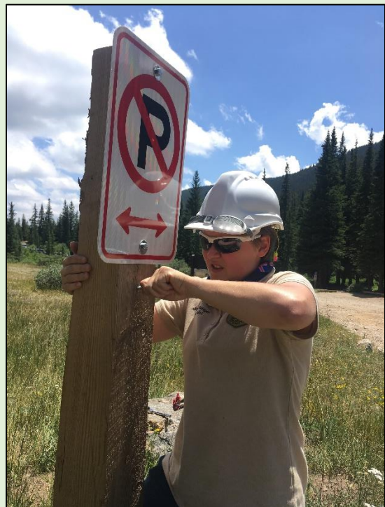
Megan installs a "No Parking" sign at the OSMP-owned 4 th of July trailhead west of Eldora, CO.
