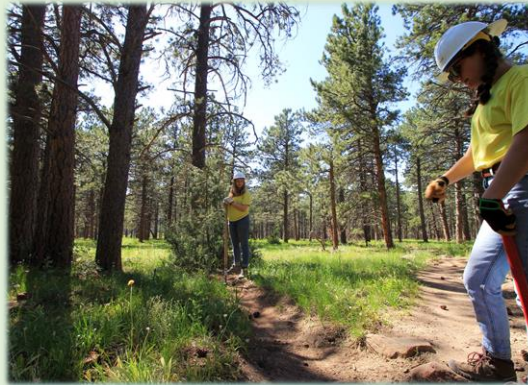
CREW 3 CLEANING AND RESHAPING THE OUTFLOW OF A ROLLING GRADE DIP ON SPRING BROOK TRAIL.
