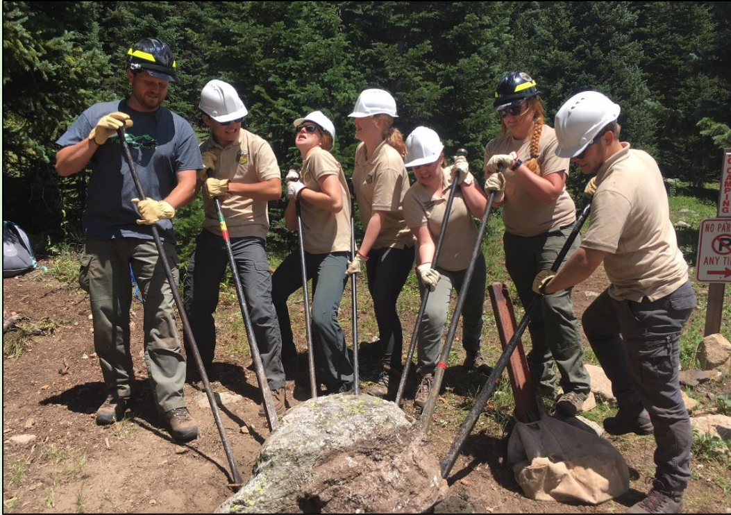
Above: Many hands make light work when it comes to repositioning large boulders at the 4 th of July trailhead.
