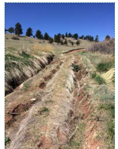
Post flood damage to legacy trail on Joder property, photo: OSMP
