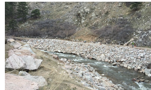
Photo 31: Bank armoring in Boulder Canyon (Reach 10)
