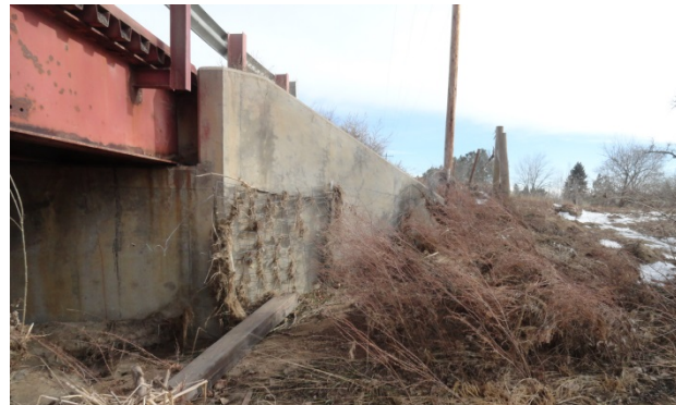
Photo 5: Flood debris at 20½ Road (Reach 2)
