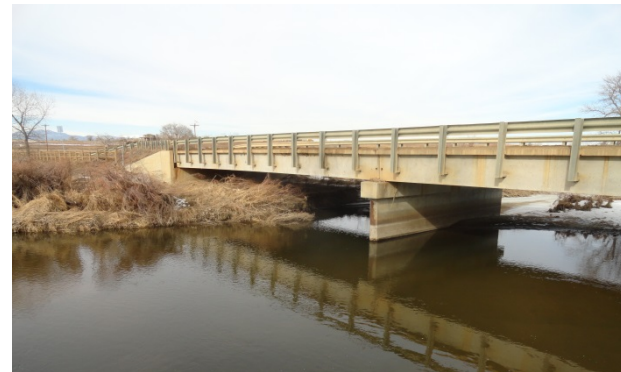
Photo 6: Pier scour at 16½ Road (Reach 2)
