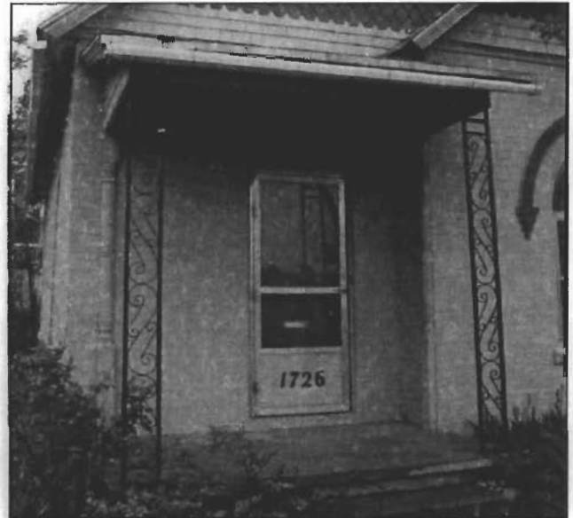
R.6: Replace the missing posts and railings when necessary. The porch posts seen above are inappropriate.
