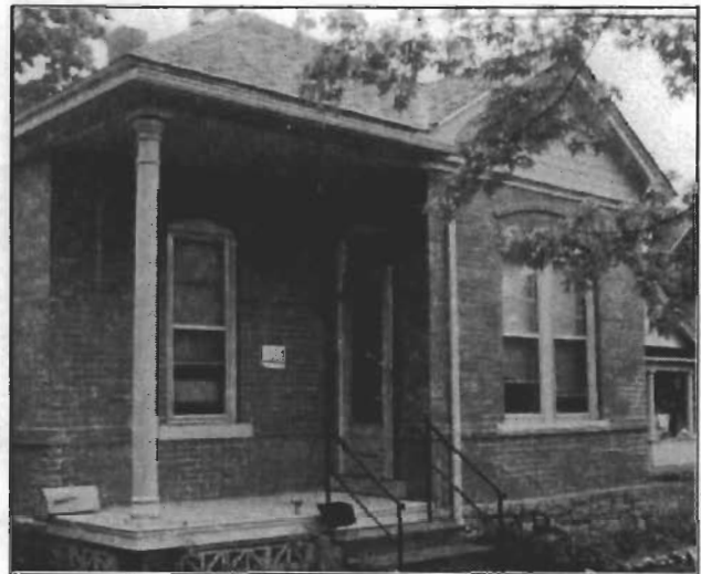
R.9: If porch replacement is necessary, reconstruct it to match the original in form and detail. The porch above is appropriate
