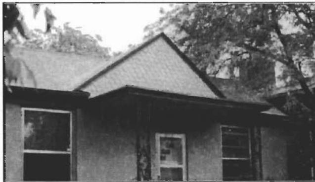
The eave depth shown above is inappropriate.
