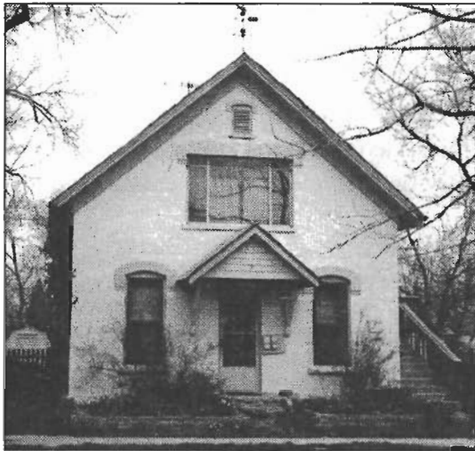
Here two windows have inappropriately been combined to create a picture window.
