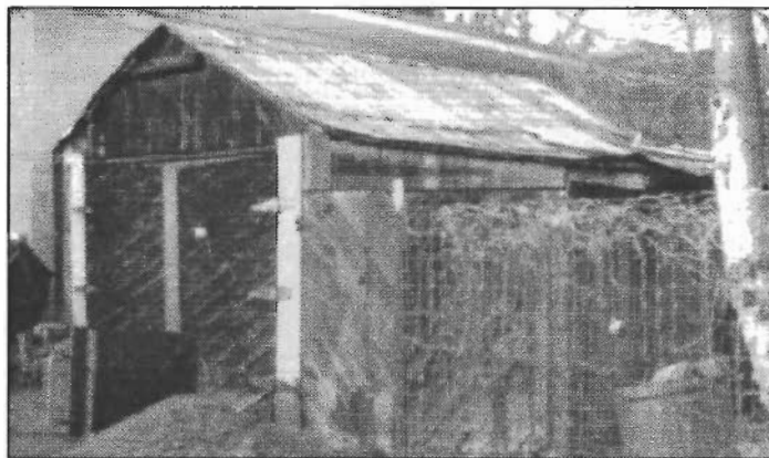
This shed, now used as a garage, retains its original historic character.
