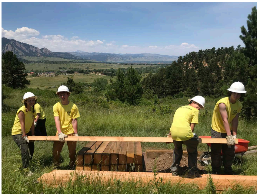
Crew 2 moving lumber to prepare for building the puncheon (bridge) on the Marshall Mesa trail
