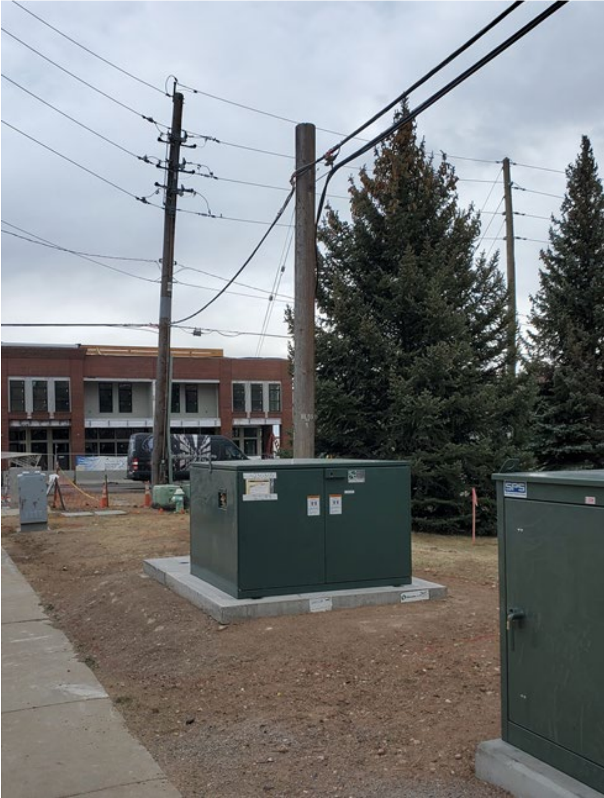
Typical Switch Cabinet:
