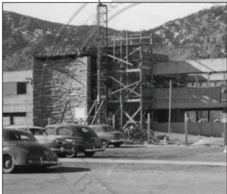
Municipal Building under construction, 1951. Photo courtesy Carnegie Branch Library for local history, Boulder Historical Society Collection.
