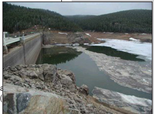
Work on the Barker Dam outlet and hydro have been deferred due to budget limitations
