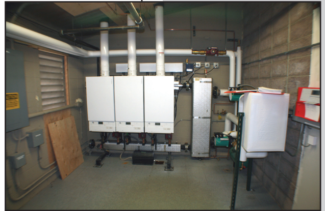
New boilers at the Spruce Pool, which when maintaining the pools temperature are 99% efficient.
